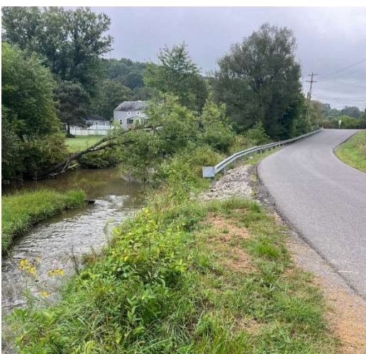
BEFORE: Dodds Road was very close to the creek, and visibility at the intersection with Rockdale Road was reduced due to the steep slope of the roadway.
